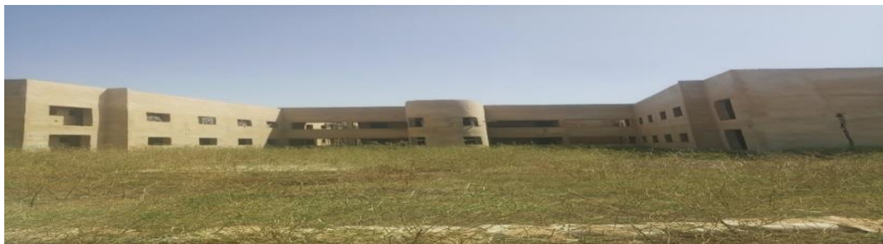
Picture 53: On-going Construction of New Operating Theatre Complex at National Orthopaedic Hospital Dala Kano
