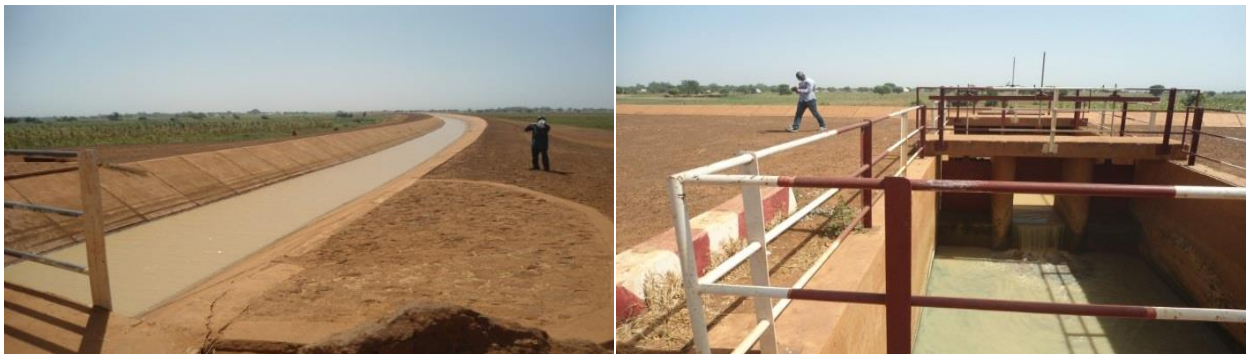
Picture 16: Completed Main Canal and its Ancillary Structures in Goronyo Dam, Sokoto State
