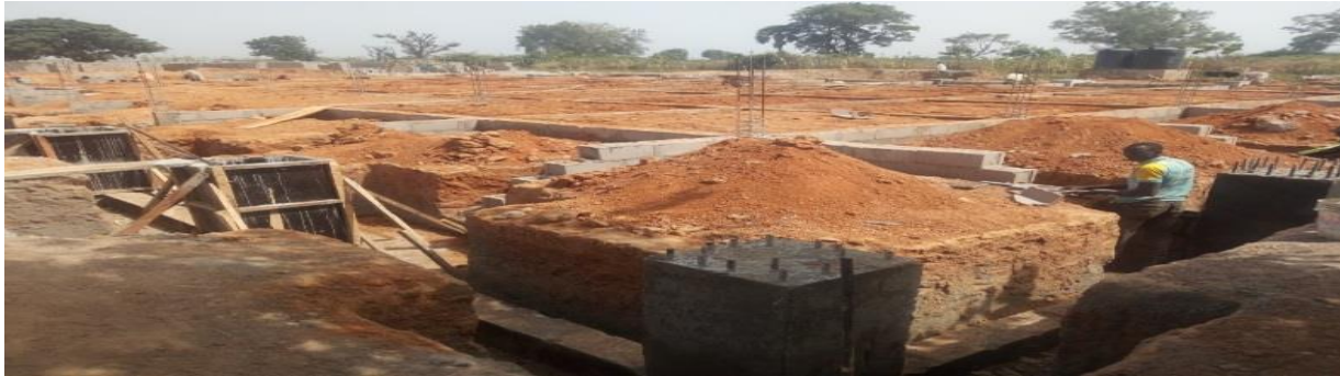
Picture 72: On-going Construction of Building for Pilot Plant for the Production of Precipitated Calcium Carbonate (PCC) at NARICT, Zaria
