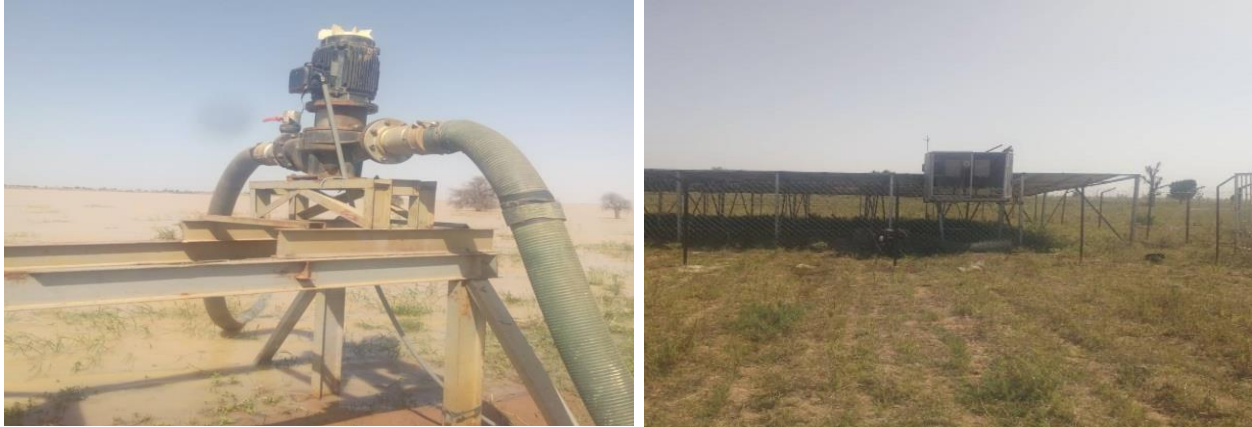
Picture 19: Installed Irrigation pump and Solar plant at the Irrigation project site
