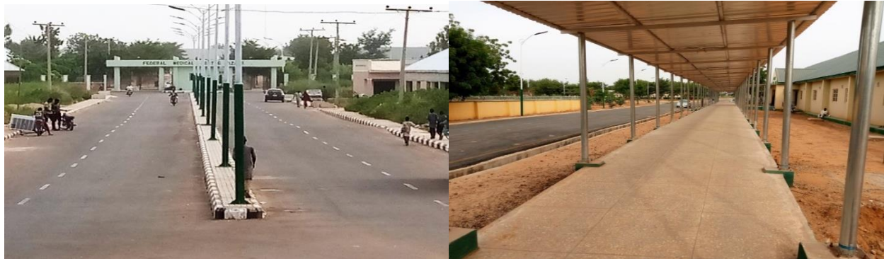
Pictures 47: Construction of Road Networks and Walk Ways at Federal Medical Centre, Azare
