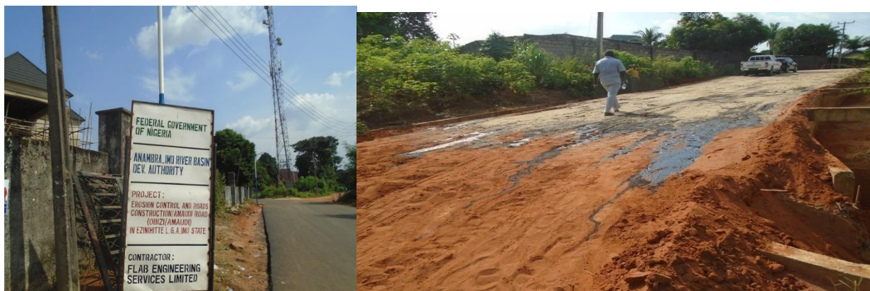
Picture 18: Erosion control and road construction at Amaudi road in Imo State
