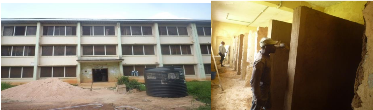
Picture 35: Construction/Renovation of the three wings old existing toilets at UNN, Enugu
