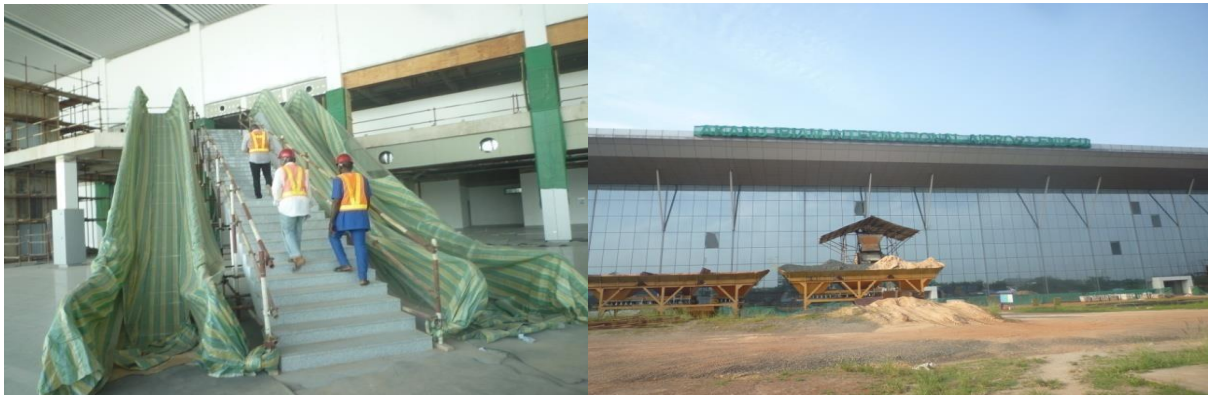
Picture 24: The installed escalators and elevators at the Terminal building of Enugu Airport
