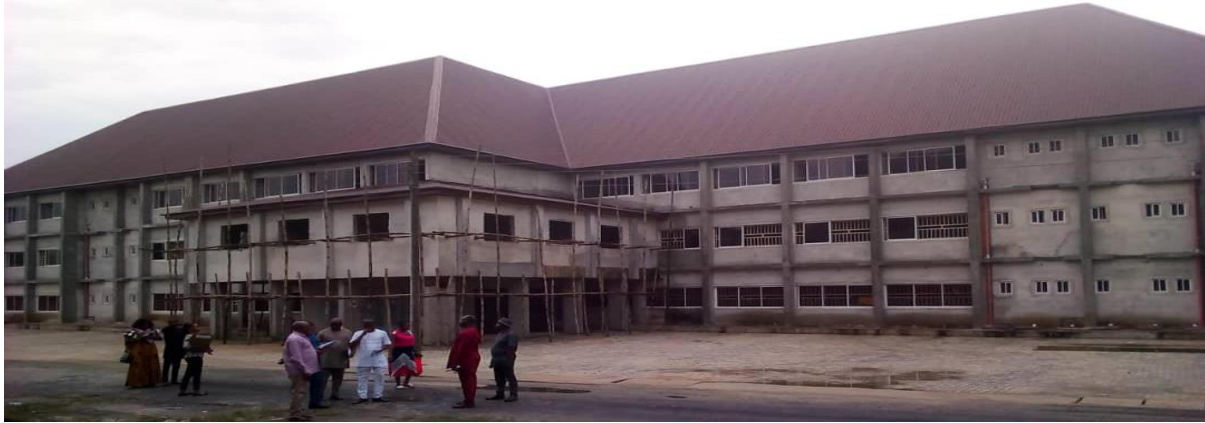
Picture 54: Ongoing Construction of Psychiatric Building at the University of Port Harcourt Teaching Hospital
