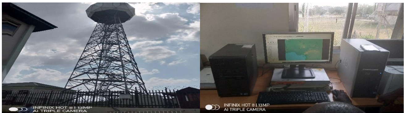
Picture 25: Installed Weather Radar and monitor
