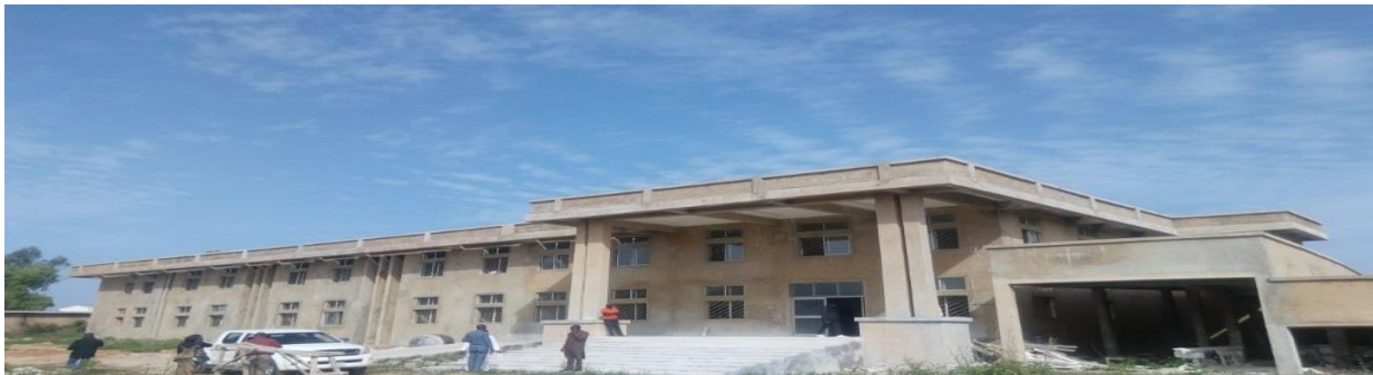
Picture 55: On-going Construction of Additional Ward (Amenity) at Jos University Teaching Hospital
