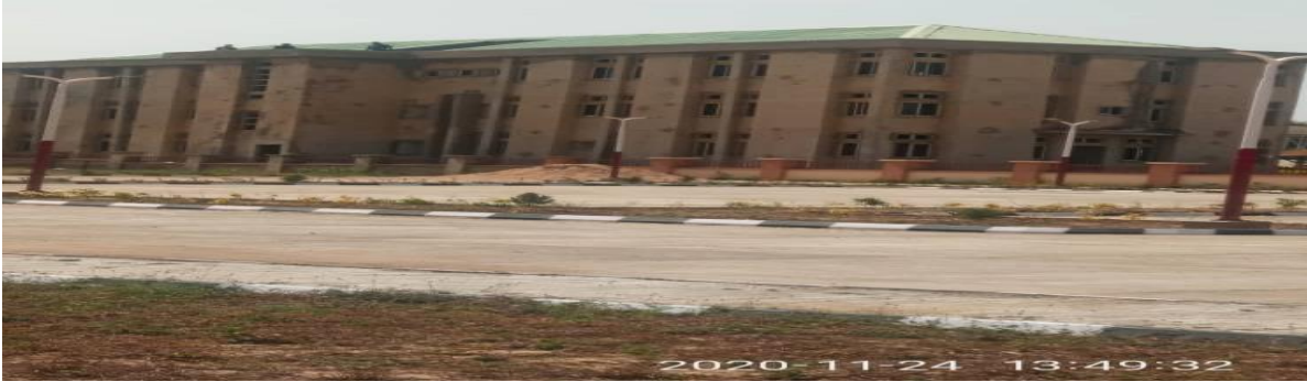
Picture 22: Ongoing construction of Director General/Chief Executive Office and Board Room at NITT Zaria
