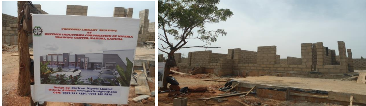
Picture 15: On-going construction and furnishing of Auditorium and Library for DICON Institute of Technology, Kaduna
