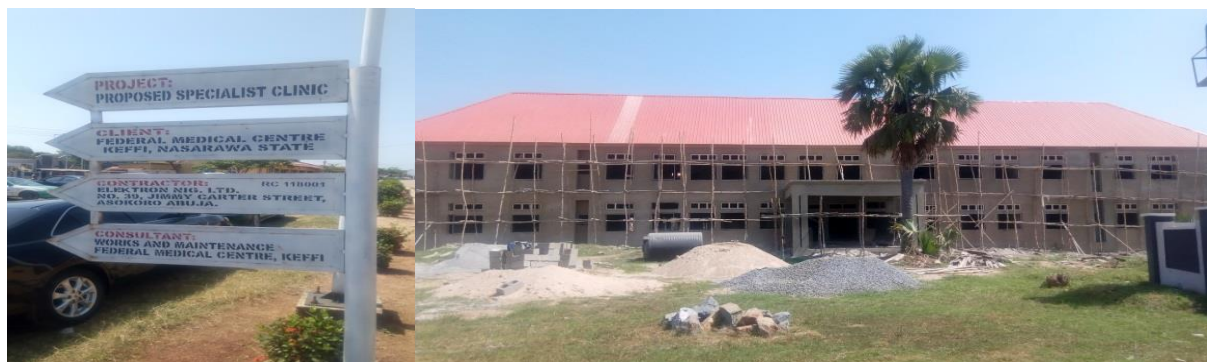
Picture 42: On-going Construction of ENT, Physiotherapy, Dental, Ophthalmology (Specialty) Patients Ward II at FMC, Keffi
