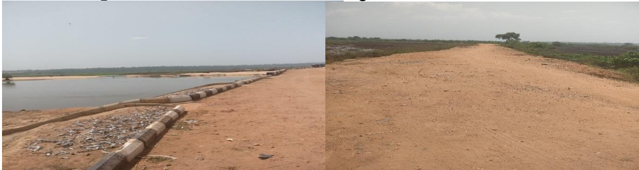
Picture 17: The completed 32km embankment (dyke) and 15km access road at Tada-Shonga Irrigation Project
