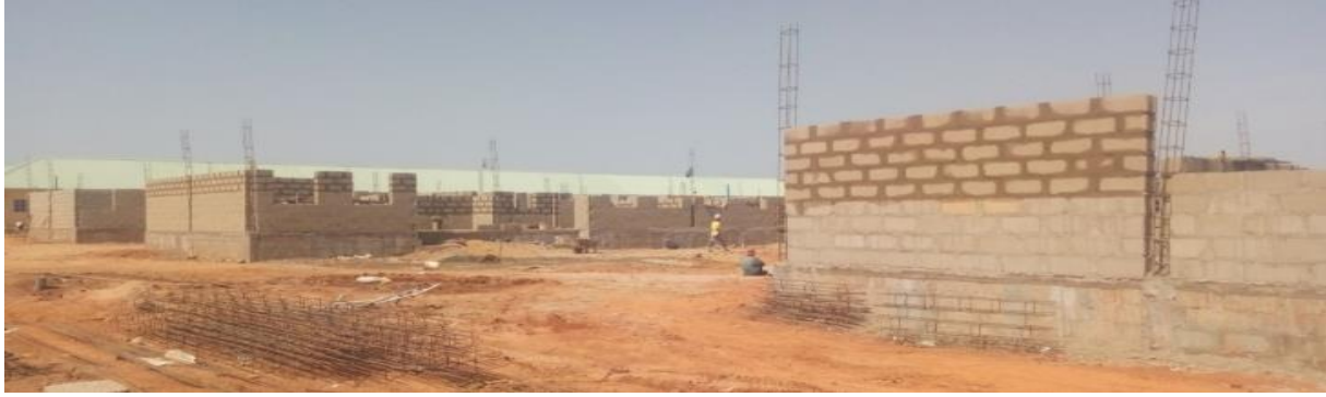
Picture 13: Ongoing Construction of 3nos Blocks of 1-Bedroom Transit Accommodation for Officers at Nigerian Defence Academy, Kaduna
