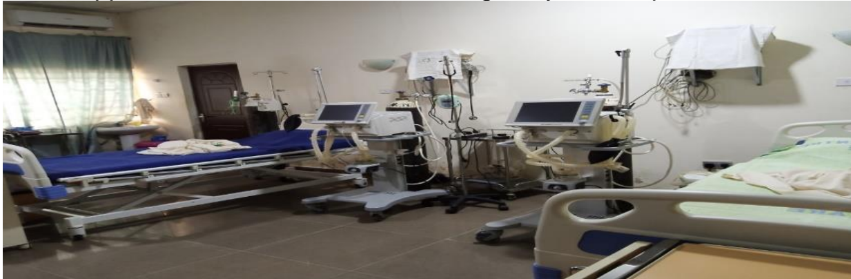
Picture 46: 2-sets of ICU Medical Equipment Installed and ready for use at FMC Azare, Bauchi State.
