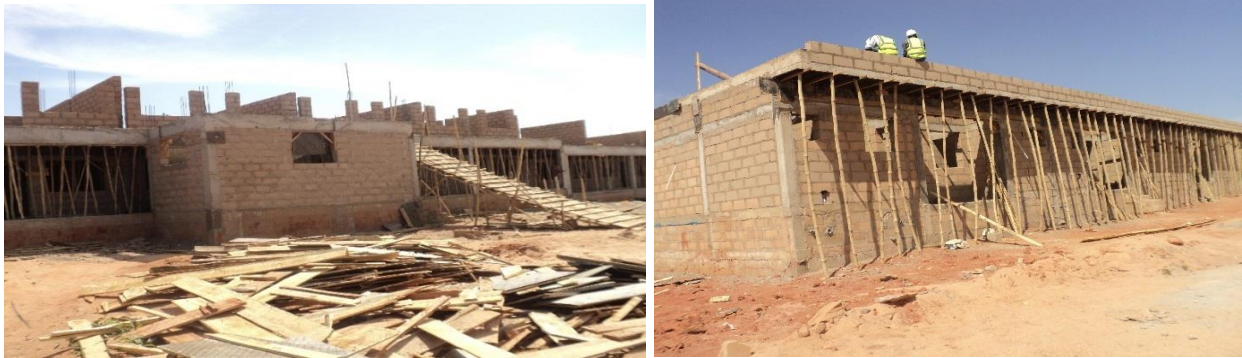
Picture 10: Construction of Transit Accommodation for Officers, Airmen and Airwomen at 175 NAF Detachment Gombe
