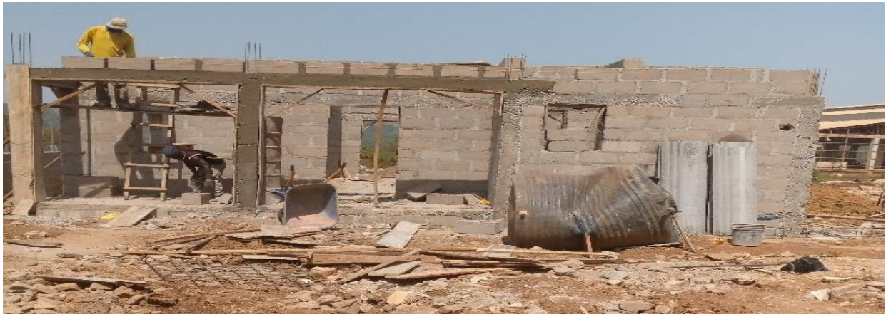
Picture 77: Ongoing construction of main gate at the National Iron Mining Project, Itakpe
