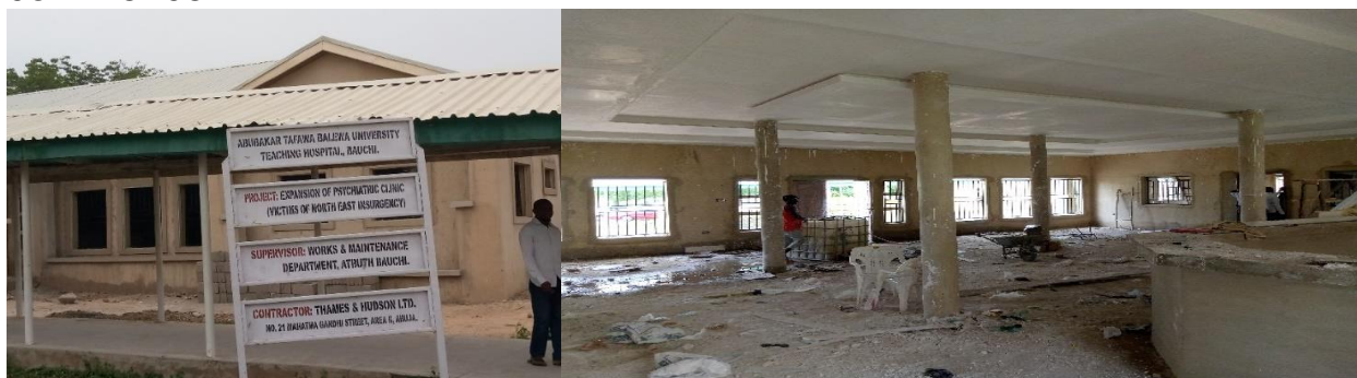
Pictures 52: Ongoing Construction of Psychiatric Clinic at the ATBU Teaching Hospital, Bauchi State
