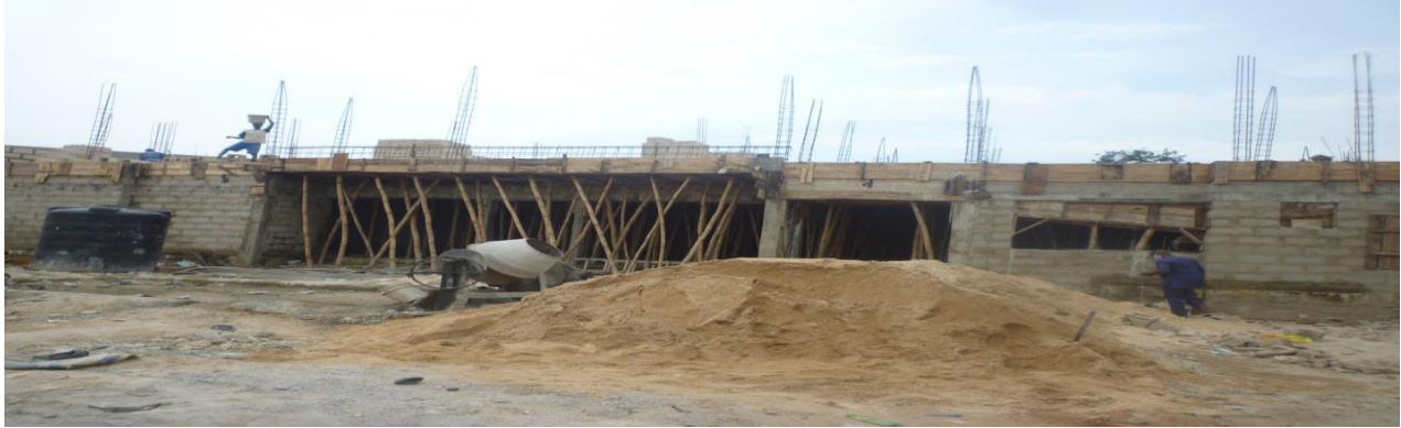
Picture 49: Ongoing works at the Accident and Emergency/ Intensive Care Unit at FMC Umuahia
