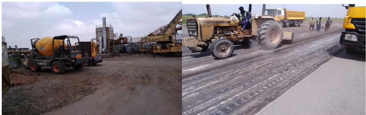
Picture 27: Extension and asphalt overlay of Runway in progress at MMIA, Lagos Airport
