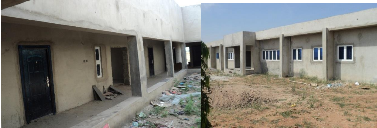
Picture 68: Construction of B.A. Gallery almost completed at the Fire Service Academy, Sheda – Kwali
