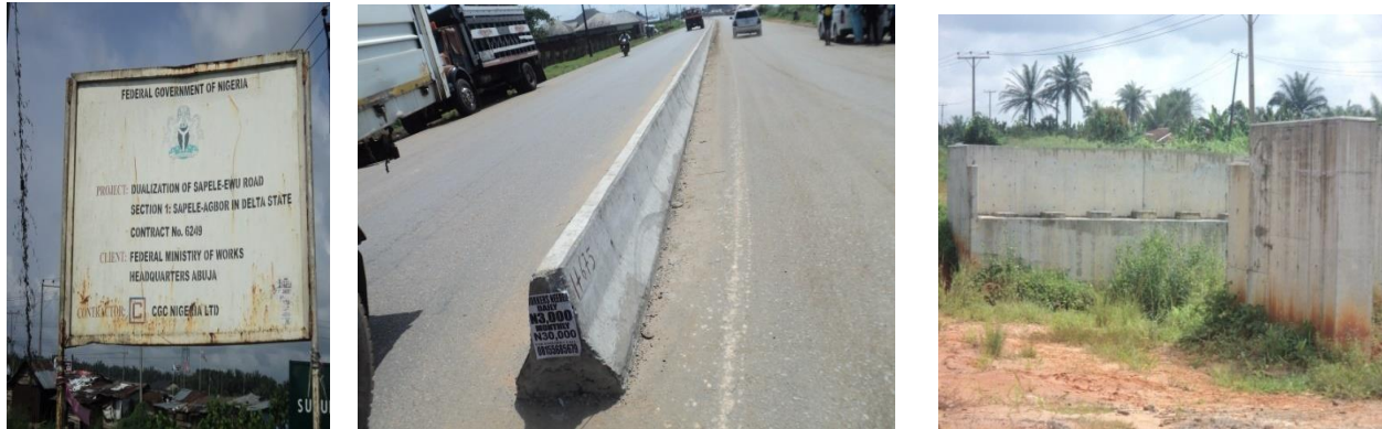
Picture 2: Completed Portions of Dualised/Single Carriage and Abutment Works at Bridge 1 (17+0.50km) around Agalokpe Community of Sapele.
