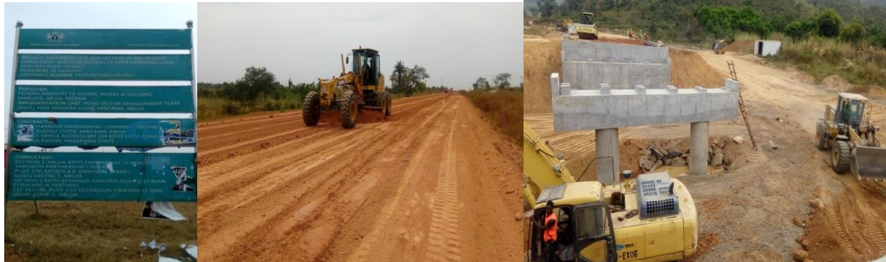
Picture1: On-going Earthworks and Bridge work between km70 – km145 (Keffi – Akwanga Axis)
