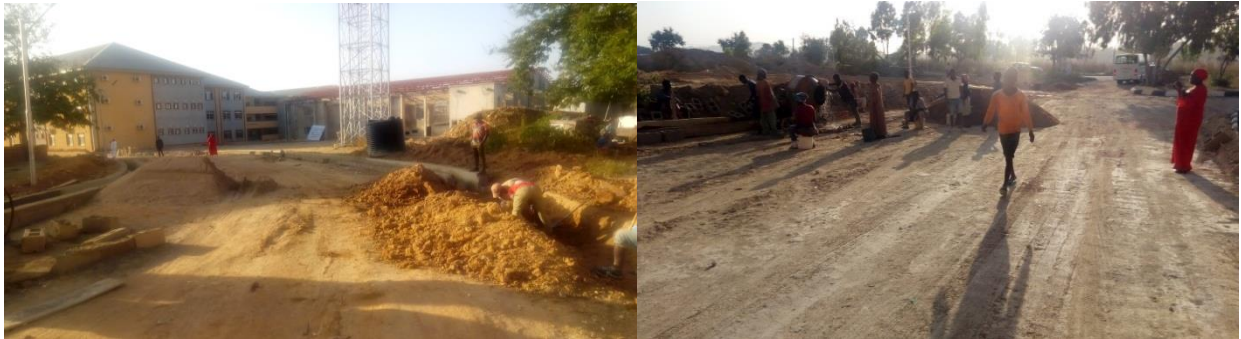
Picture 31: On-going construction of internal access road at the University of Jos
