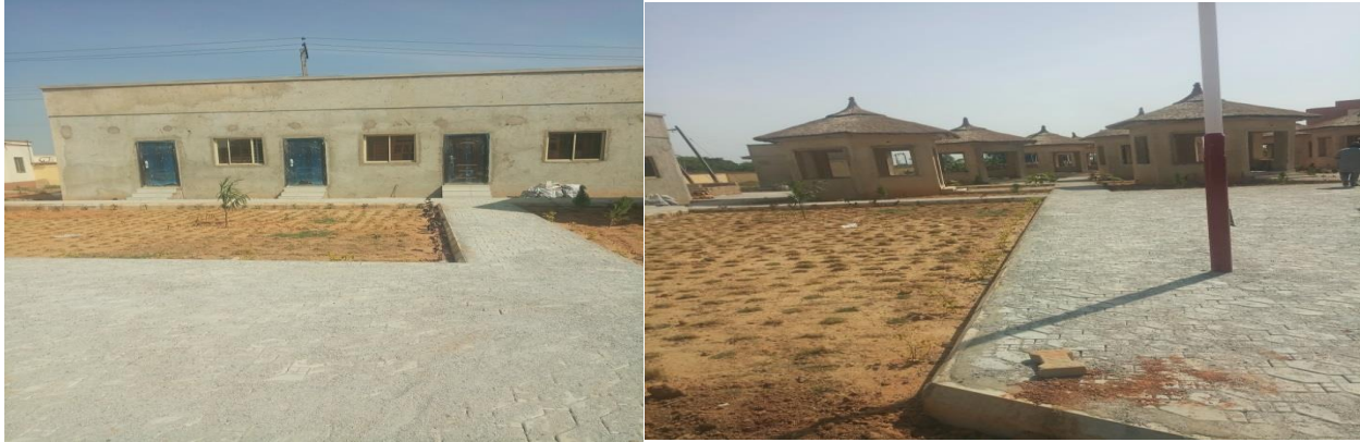
Picture 23: Ongoing construction of Garden and Parks Development, Landscaping and Upgrading of Lighting System
