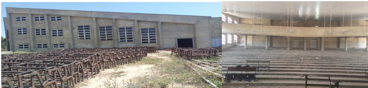
Picture 38: On-going Construction of 1,500 Seating Capacity Lecture Theatre at Federal College of Education Zaria
