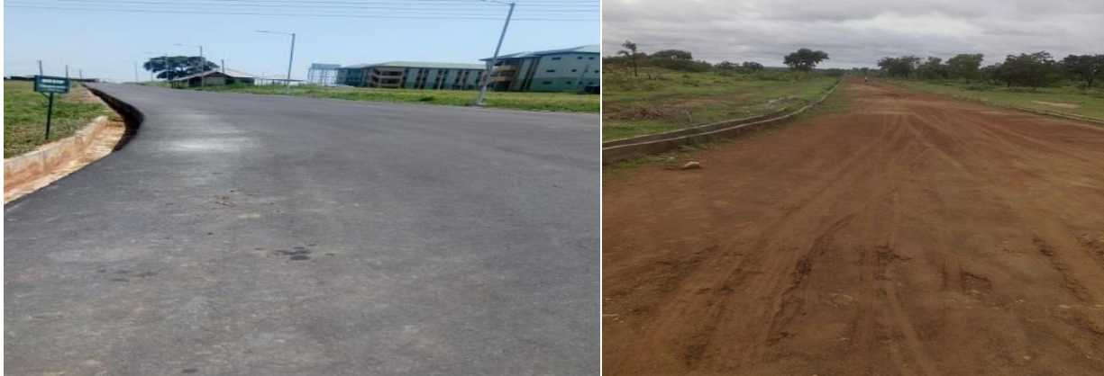
Picture 56: A Section of the Completed Asphaltic Access Road Network and the Ongoing Graded Portion of the Road at University of Agriculture, Makurdi
