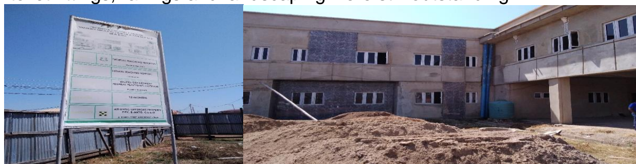
Picture 51: On-going Construction of Modern Accidents and Emergency Building at FTH Ido-Ekiti
