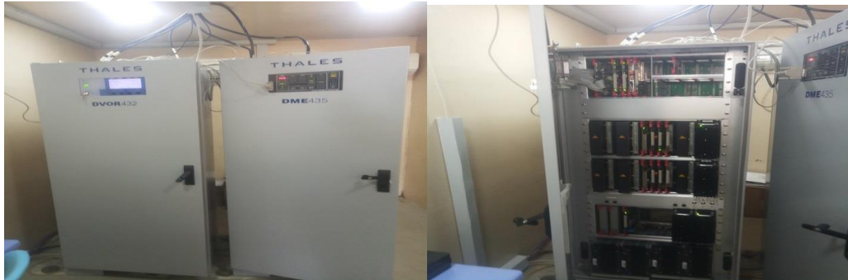
Picture 29: Installed DVOR/DME and ILS at NCAT, Zaria
