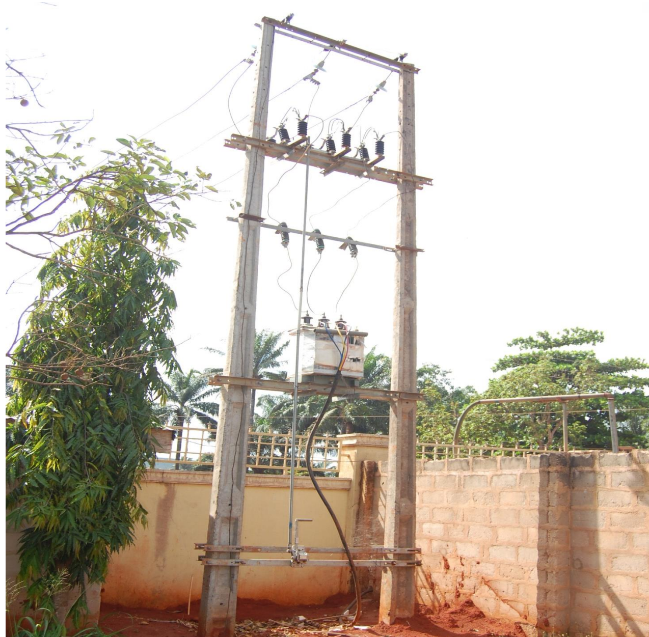
Extension of Electricity to Zik's Flats Nsukka with 100KVA, 11/0.415 Distribution Transformer
