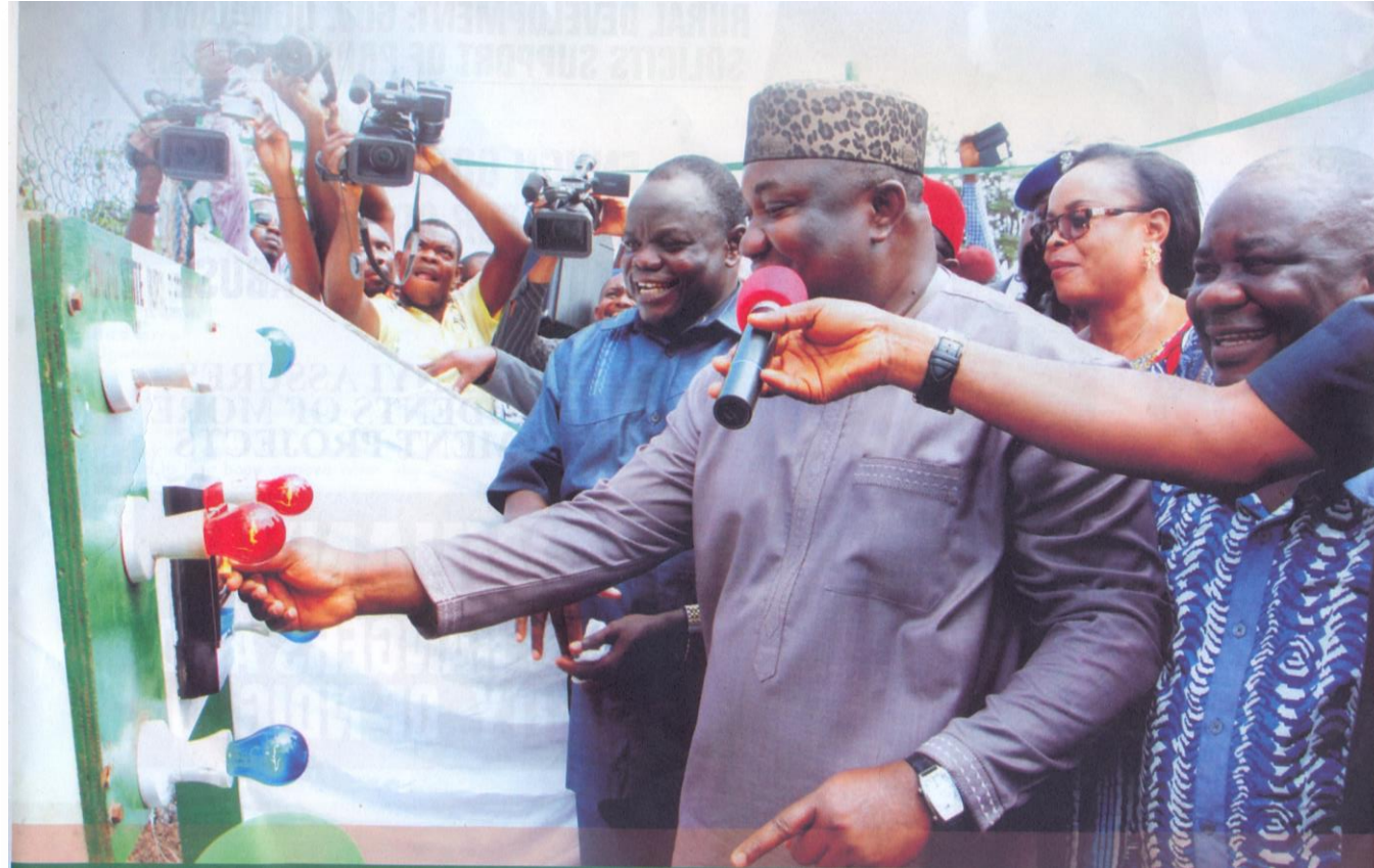
Inauguration of 15KM Inter-Town Connection (ITC) 2.5 MVA Injection Sub - Station at Ezi-Nze, Udi Local Government Area by His Excellency, Rt, Hon. Ifeanyi Ugwuanyi, governor, Enugu State
