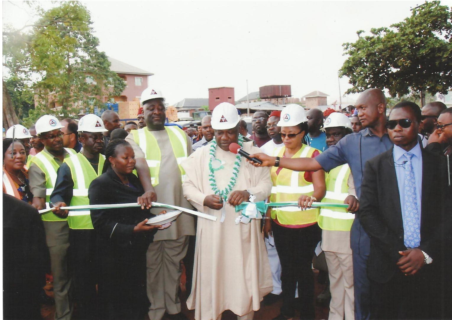
Flag-Off of the Construction of Nsukka Urban Roads by His Excellency, Rt. Hon. Ifeanyi Ugwuanyi, Governor, Enugu State
