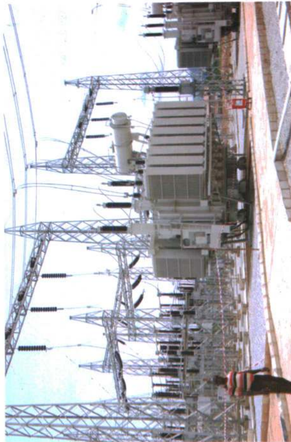
Newly Installed Power Sub-Station in Lafia.
