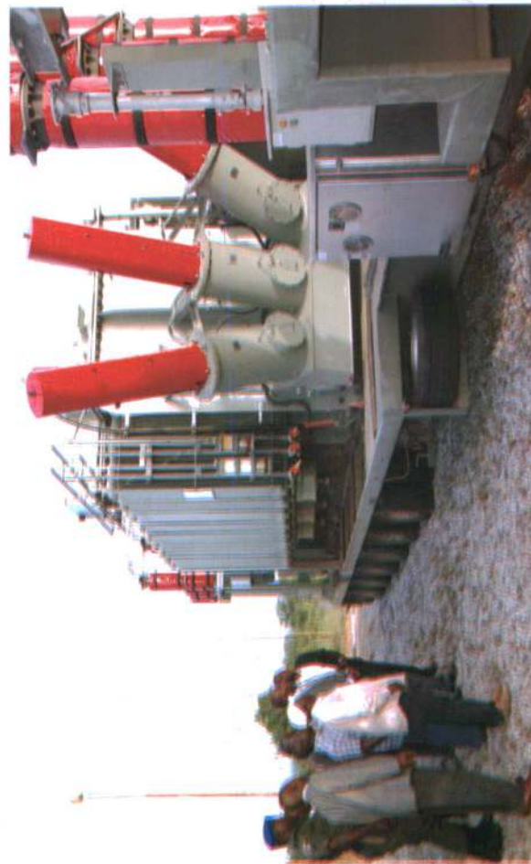
Gov. Umaru Tanko Al-Makura Inspecting 60 MVA Transformer at Akwanga Sub-Station
